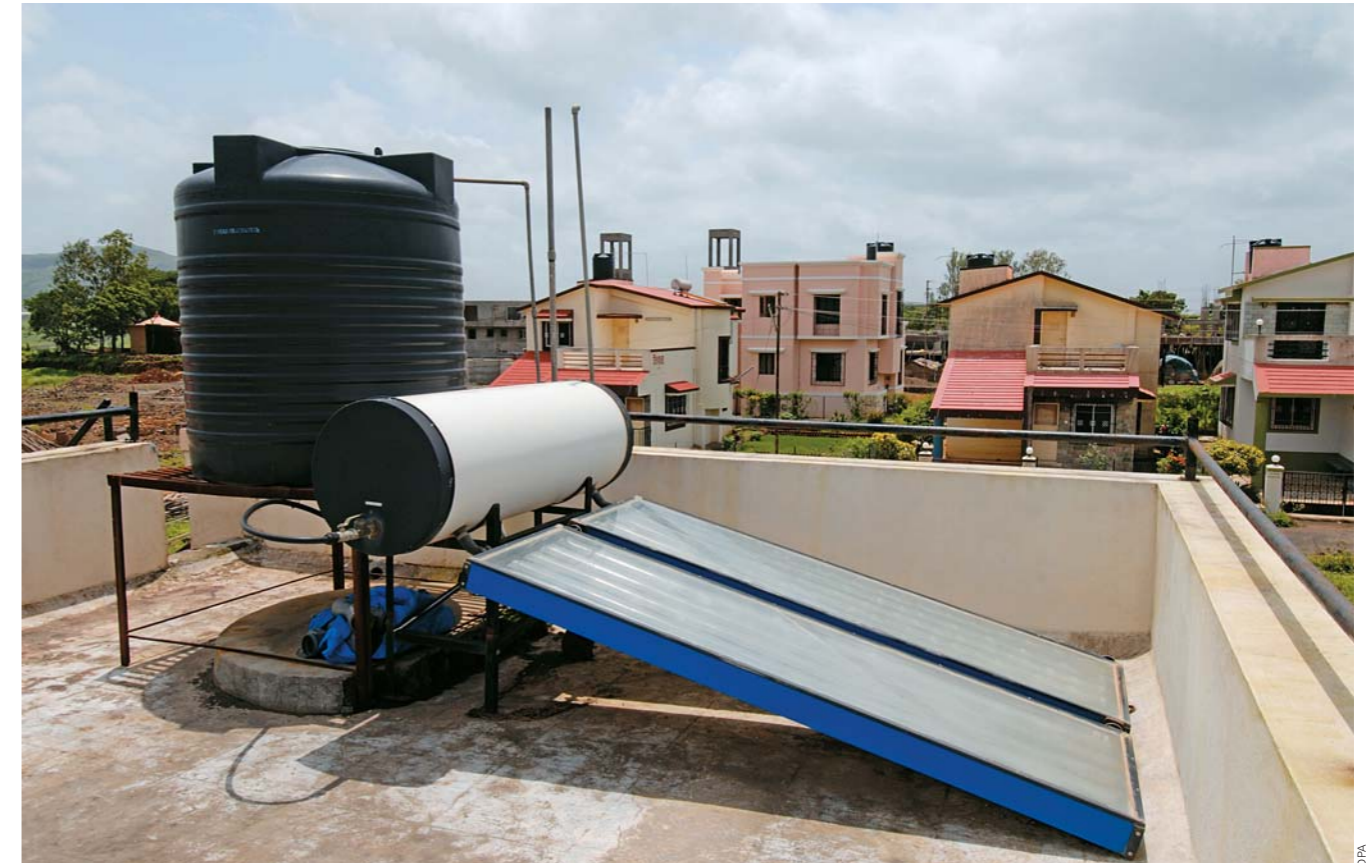
WHAT-A HEATER: About 2.15 million sq m of collector area has been installed in India for solar water heating applications
